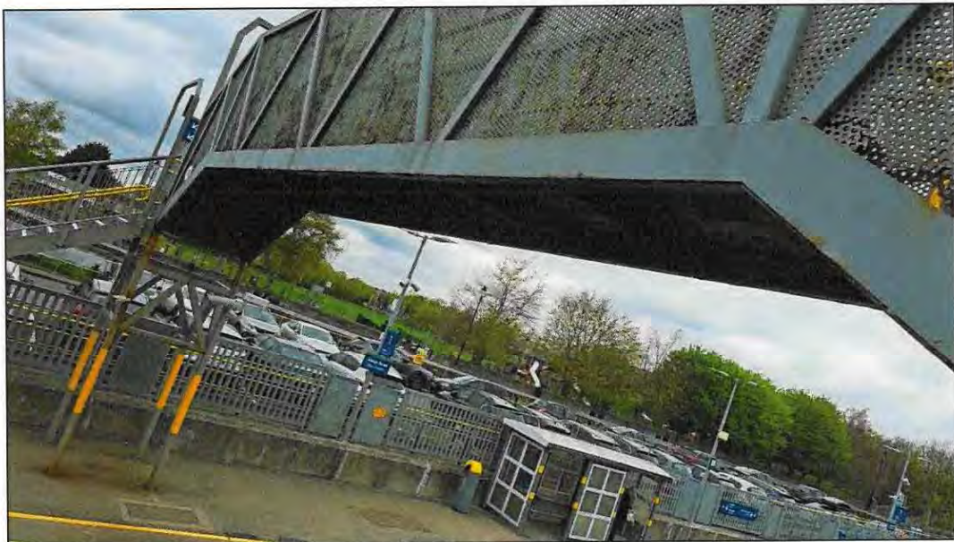
Plate 5-7 Underside of existing bridge, which does not provide suitable habitat for roosting bats
